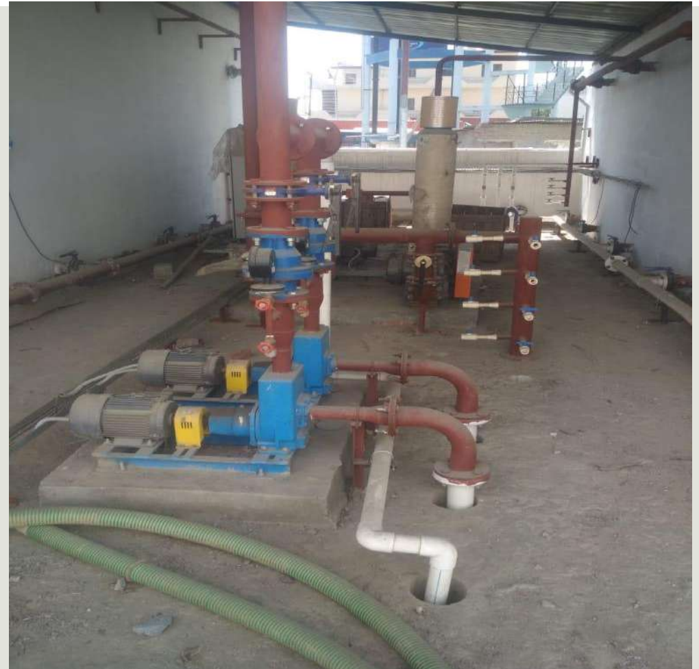
STP at AHP Transport Nagar Dehradun
