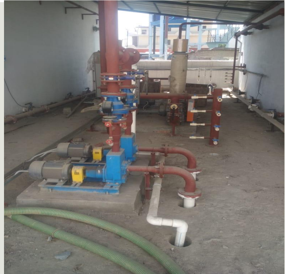
STP at AHP Transport Nagar Dehradun
